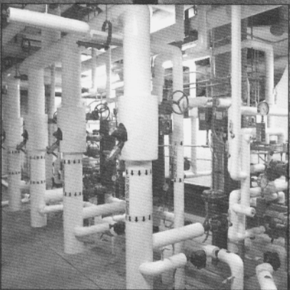
Semi-instantaneous, steam-heated hot water heater.
