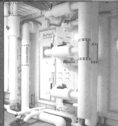
One of the building's six large air-handlers.
