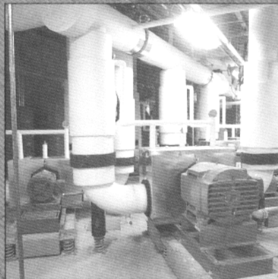
Primary and backup pump circulates chilled water throughout the building.
